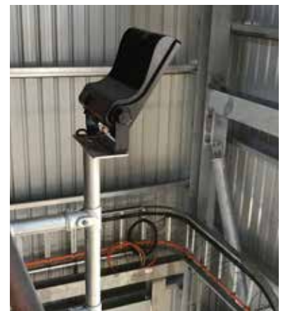
LED Light Fittings Fitted to Poles
