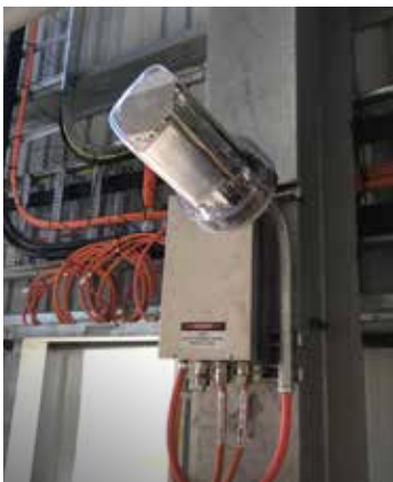
Junction Boxes Fitted with Terminals and Gland Entries
